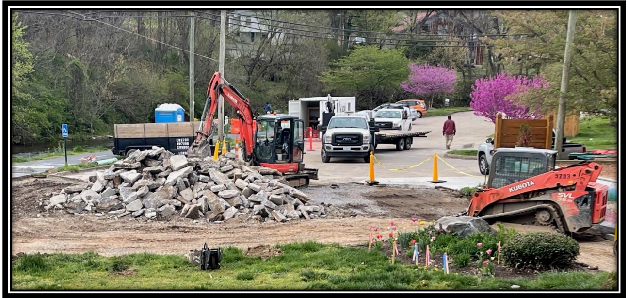
The Ruffner Plaza concrete area is being replaced due to safety issues. The grass will remain, and the benches will return after construction.
