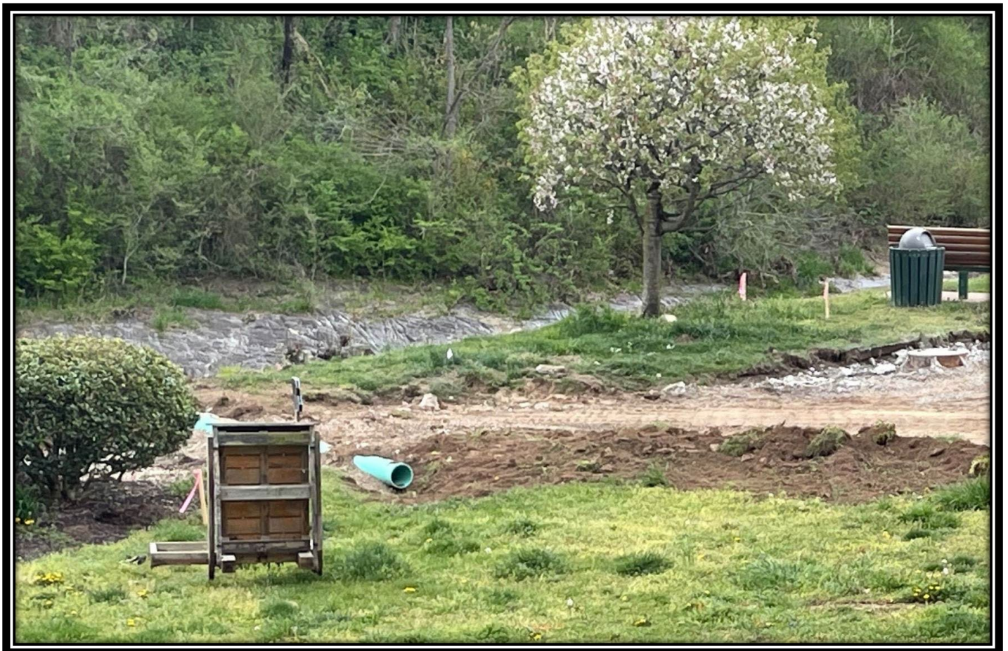
The grass and concrete drainage are being improved for safety and longevity.
